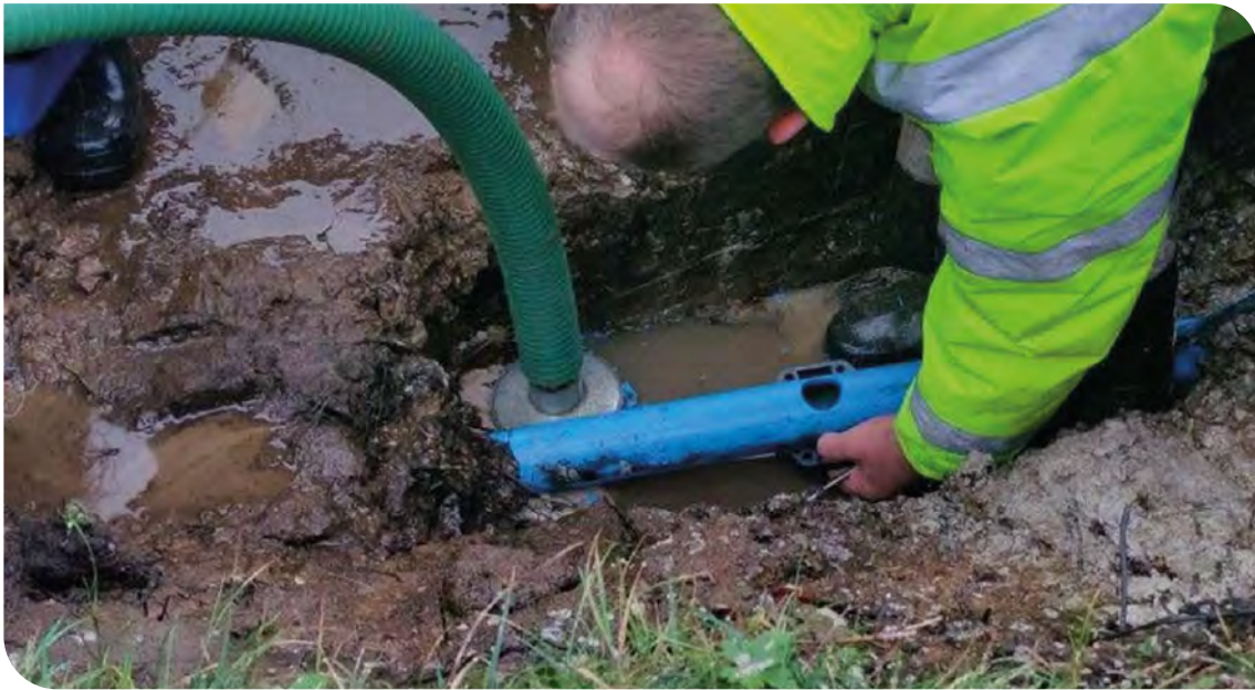
The fibre cable is delivered through a second pipe housed within the drinking water network
